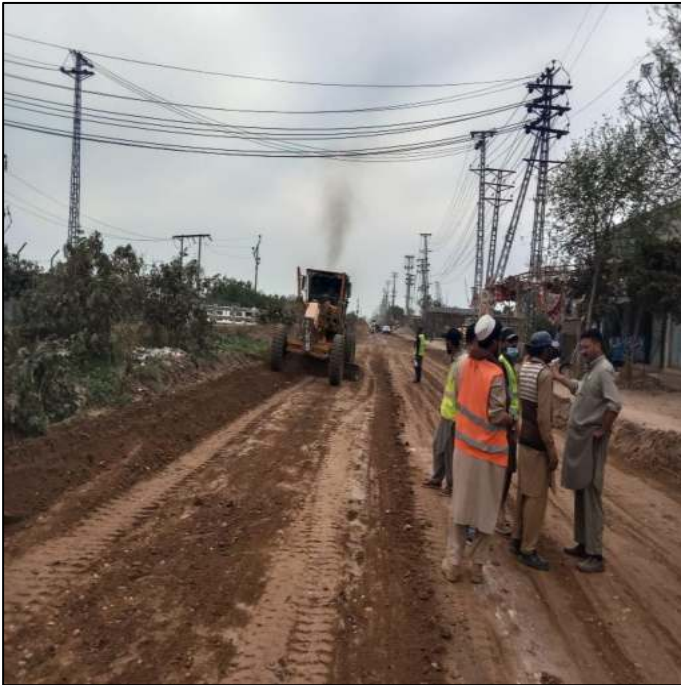
Picture 35: Restoration of Airport Road up to Sub Grade Level is in Progress
