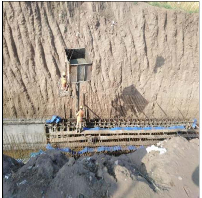
Picture 16: Concrete Pouring through Tremie Pipe at Box Conduit (7'x6.5') is in progress
