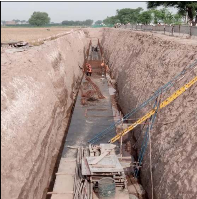
Picture 15: Construction of RC Cast In-Situ Box Conduit (7'x6.5') is in progress
