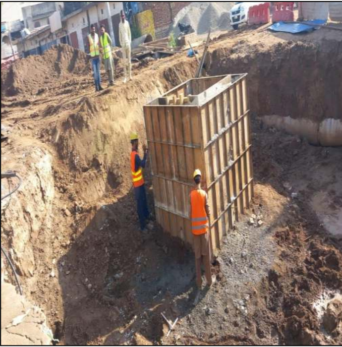
Picture 27: Lot-02: Shaft Formwork Opening Manhole No. 50 in Progress at Marala Road
