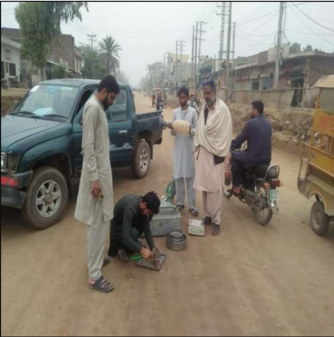
Picture 29: Lot-02: FDT in Progress at Sub Grade Top at Airport Road
