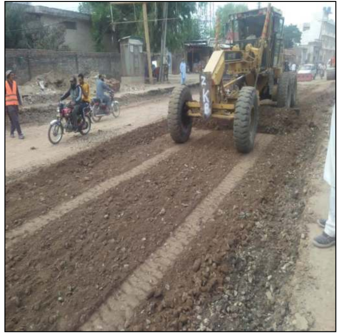
Picture 28: Lot-02: Sub Base Grading and Mixing in Progress at Marala Road
