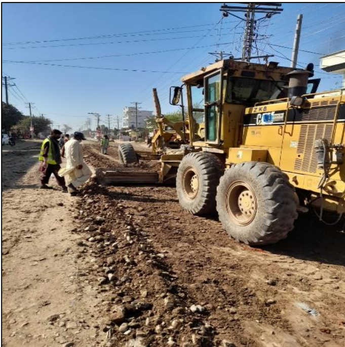
Picture 37: Gradation of Sub Base 1st Layer is in Progress at Airport Road
