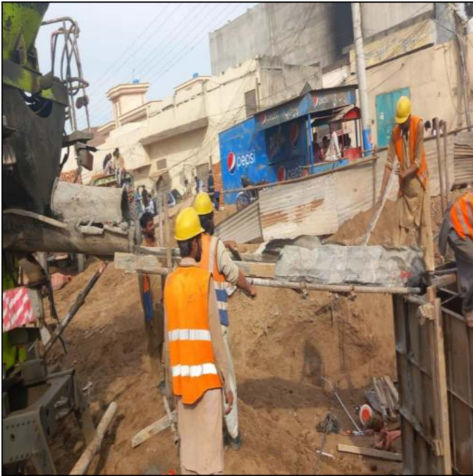
Picture 31: Lot-02: Shaft Wall Concrete Pouring in Progress Manhole 45 at Marala Road
